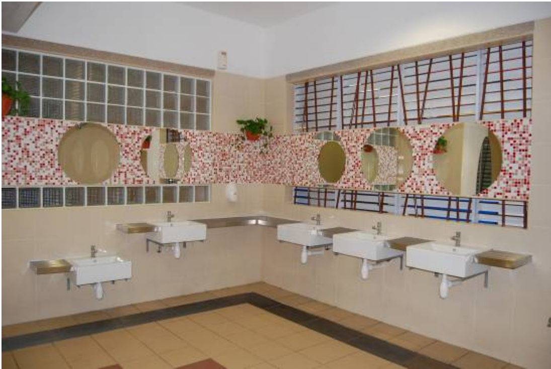
Entrance and interior of the 5-star public toilet at Blk 162 Ang Mo Kio Ave 4
